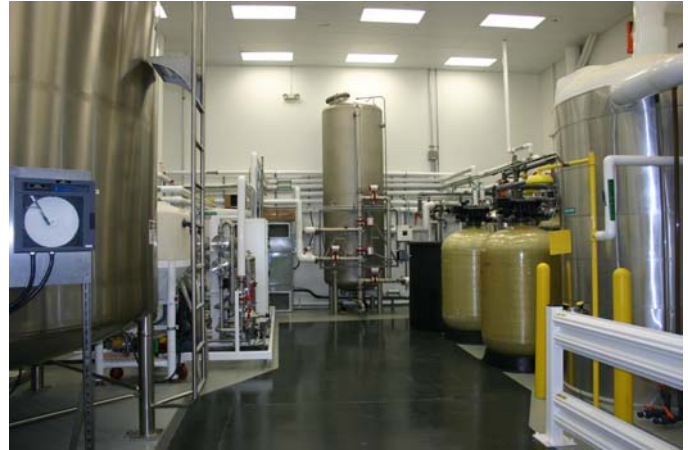
Purified Water System
